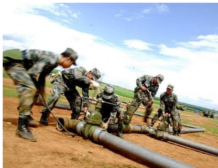
Fig 1. Field oil pipeline
