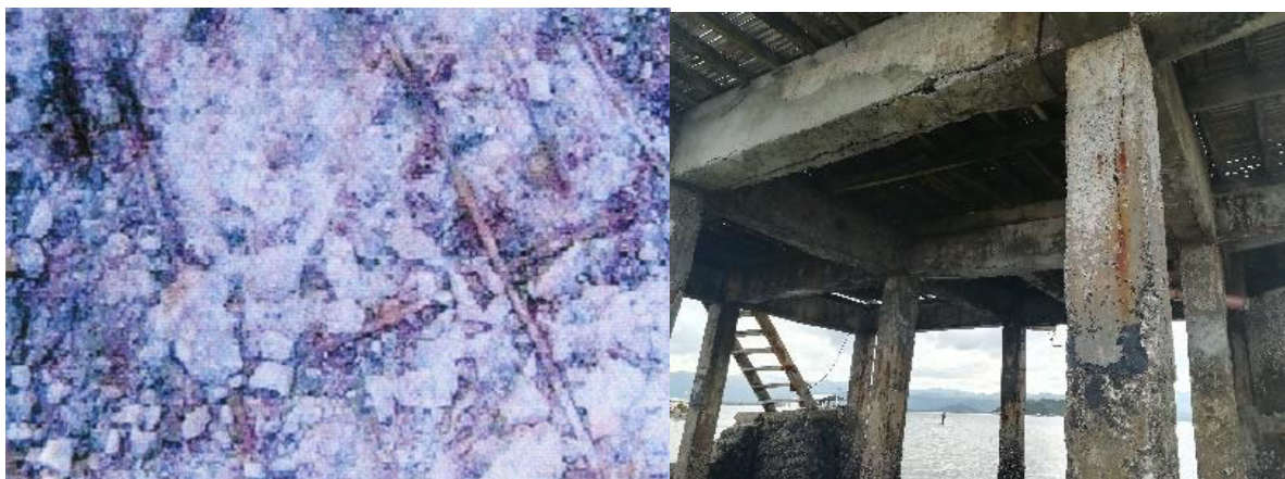
Figure 1. Example of chlorine salt erosion under freeze-thaw cycle in north China
